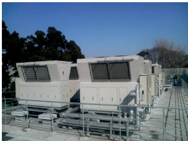
Figure 9. New chillers with hermetic ammonia scroll and conventional condensers.
